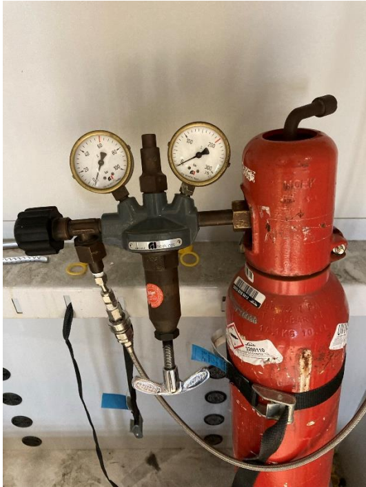
Figure 18: Metal hose connected to the gas cylinder
